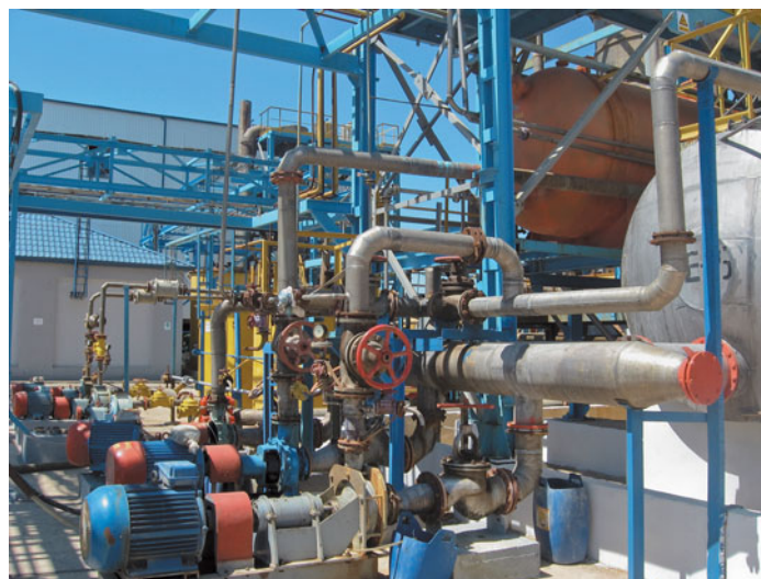
FIGURE 1.1 Industrial and commercial fluid piping systems, like this one used in a chemical processing plant, involve complex arrangements requiring careful design and analysis. (Source: Nikolay Kazachok/Fotolia)
